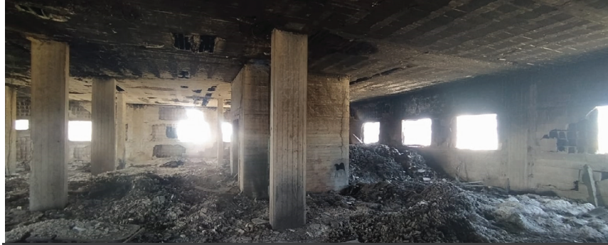
Pictures of the damage sustained by the Hind Daghma Dialysis Center which will be rebuilt through the collaboration with UOSSM.
